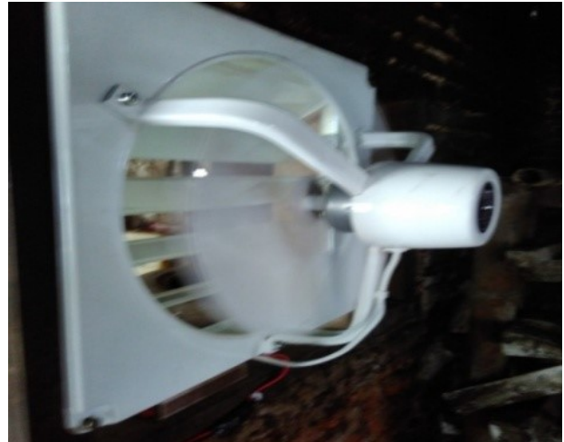
Picture 4. Exhaust fan.
