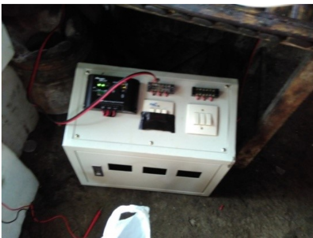
Picture 3. Charge Controller. Battery in One Box.
